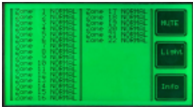
Normal, no alarm or faults
